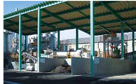
SRP Mixes insolubilizer into inorganic matter sludge, then granulates and fires it to be used in recycled items.
