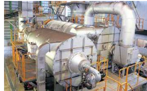
AKT Combusts distillation gas from the carbonizing process. Its self-carbonizing system helps it consume almost no fossil fuel.
